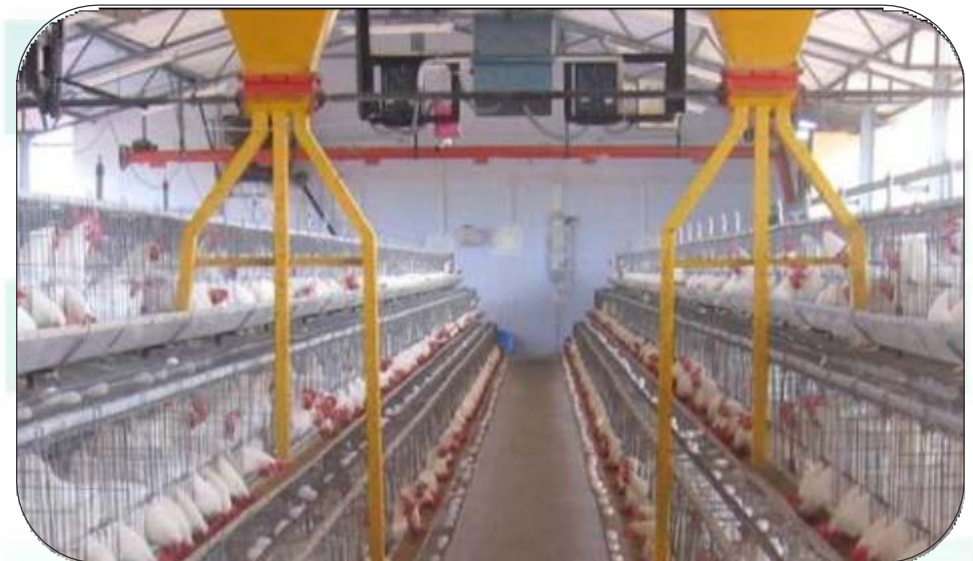
Project Name : Venco Research and Breeding Farm Pvt. Ltd. Client : Venco Research and Breeding Farm Pvt. Ltd. Description Electrical allied infrastructure works for Factory Building at Shirval.
